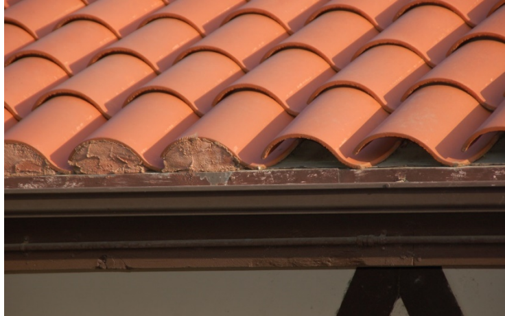
Figure 6.6. Use of a mortar mix to provide an effective “bird stop” at the edge of this barrel style roof (this photograph was taken during a retrofit project while the work was in progress). Photo: Stephen L. Quarles
