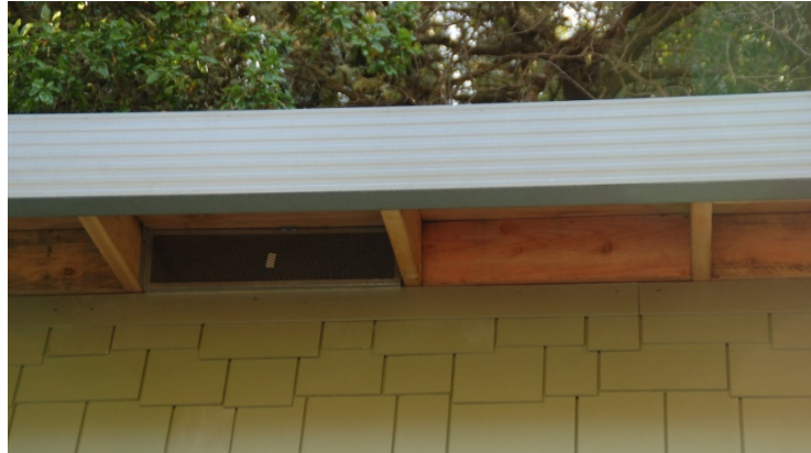
Figure 6.3. Vent located in the blocking space in open-eave construction. Photo: Stephen L. Quarles
