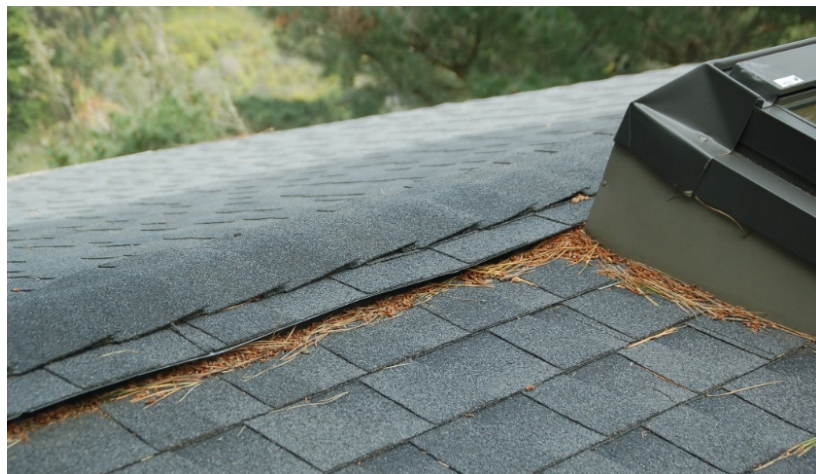
Figure 6.2. Debris accumulation at the entry of a (plastic) ridge vent. Ember ignition of this debris could result in ignition of the ridge vent. Photo: Stephen L. Quarles
